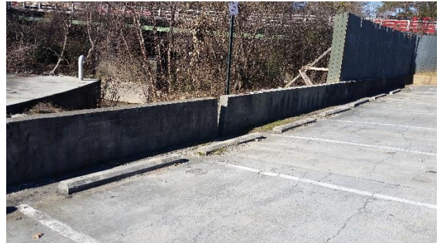
Figure 2-17. Example of a Non-Functional Stormwater Management Structure Needing Maintenance
