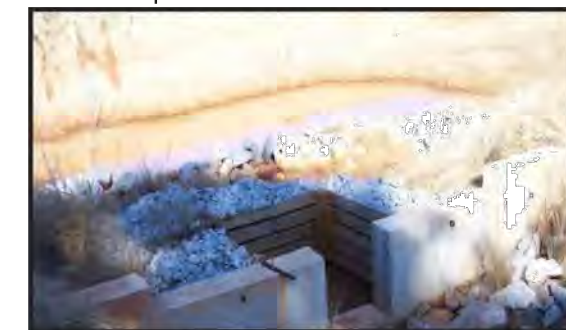
Example of Slotted Board Dam
